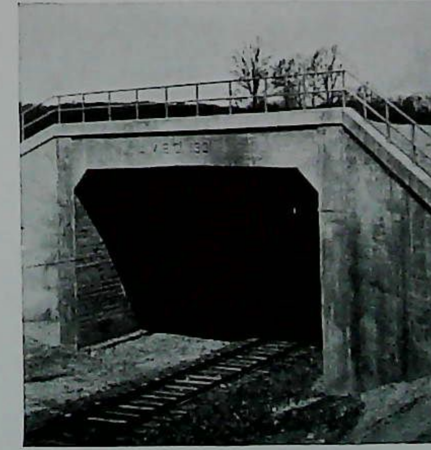
Bridge and Underpass, Washington, D. C. Waterproofed with Barrett materials. Fabric used on top and sides
